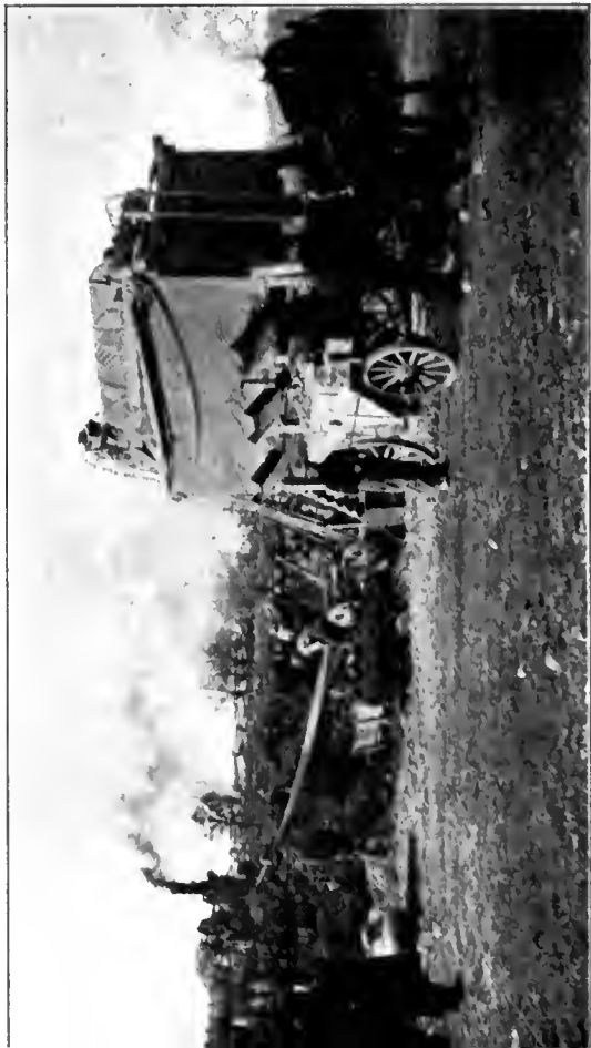
Arrangement of Crushing Equipment—Stone carried from the quarry face in small cars operated over portable steel tracks.
